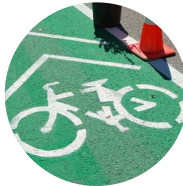
T&D painted temporary Shared Lane Markings (sharrows) on the streets during the Street Smart demonstration weekend. source: CPEX
