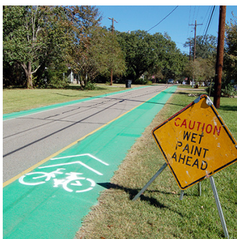
Bike lanes on Capital Heights Avenue were painted to increase visibility and safety.
