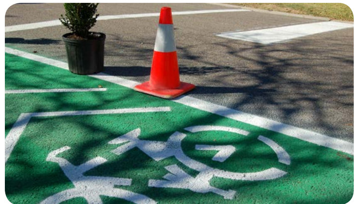
One of the temporary installations that was tested during the demonstration weekend
