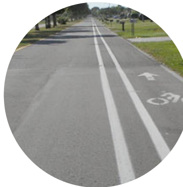
Buffered bike lane in a residential area of Cape Coral, FL, where simple solid white lines are used when the buffer zone is less than three feet wide. source: NACTO
